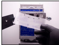
2. The oil mist detector needs to be in operation mode with negative pressure set to 60mmWC.
